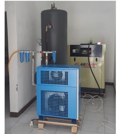
Compressor, Air Tank & Jet Mill Filter
